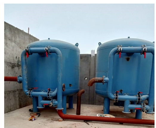
Pressure Sand Filter (FRP-MSEP)
