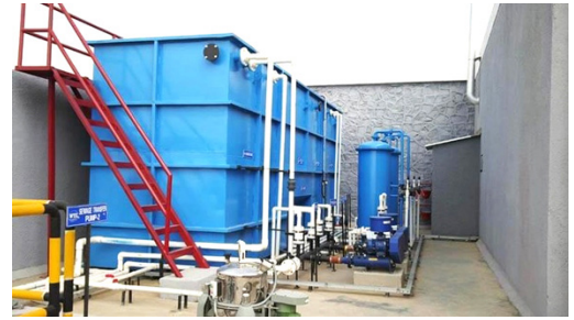
Packaged STP Plant (MSEP)
