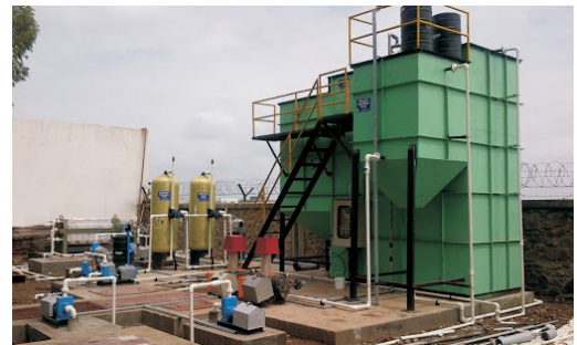
Packaged ETP Plant (MSEP)
