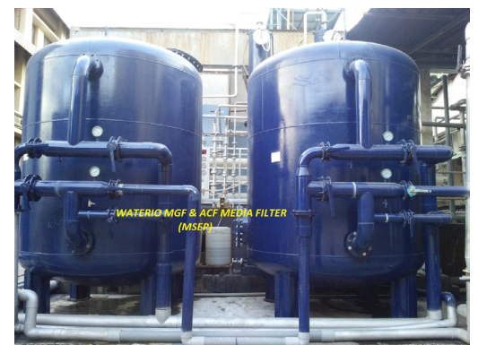
Activated Carbon Filter (FRP-MSEP)
